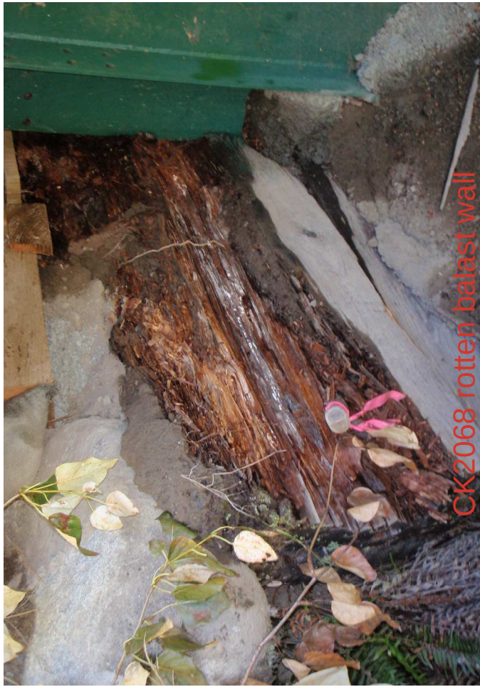
CK2068 Right abutment rotten tie backs
